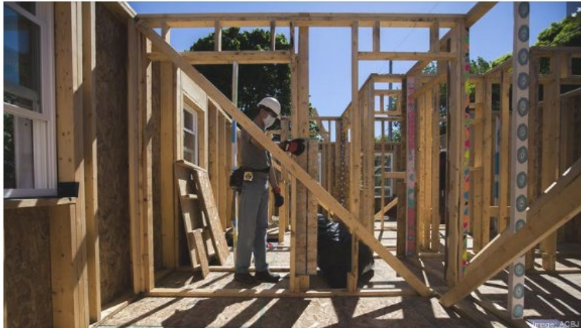
Milwaukee Habitat for Humanity and Emem Group were selected to build 120 houses and duplexes in Milwaukee's King Park neighborhood. KENNY YOO/MBJ
