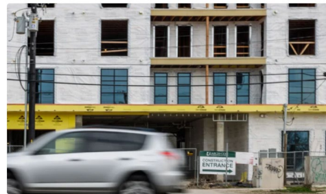
Photo by Julius Shieh/ KUT News. Nearly 400 apartments are under construction in a new building on Burnet Road. Developers began building a record number of apartments in the first years of the pandemic, many of which are opening now.
